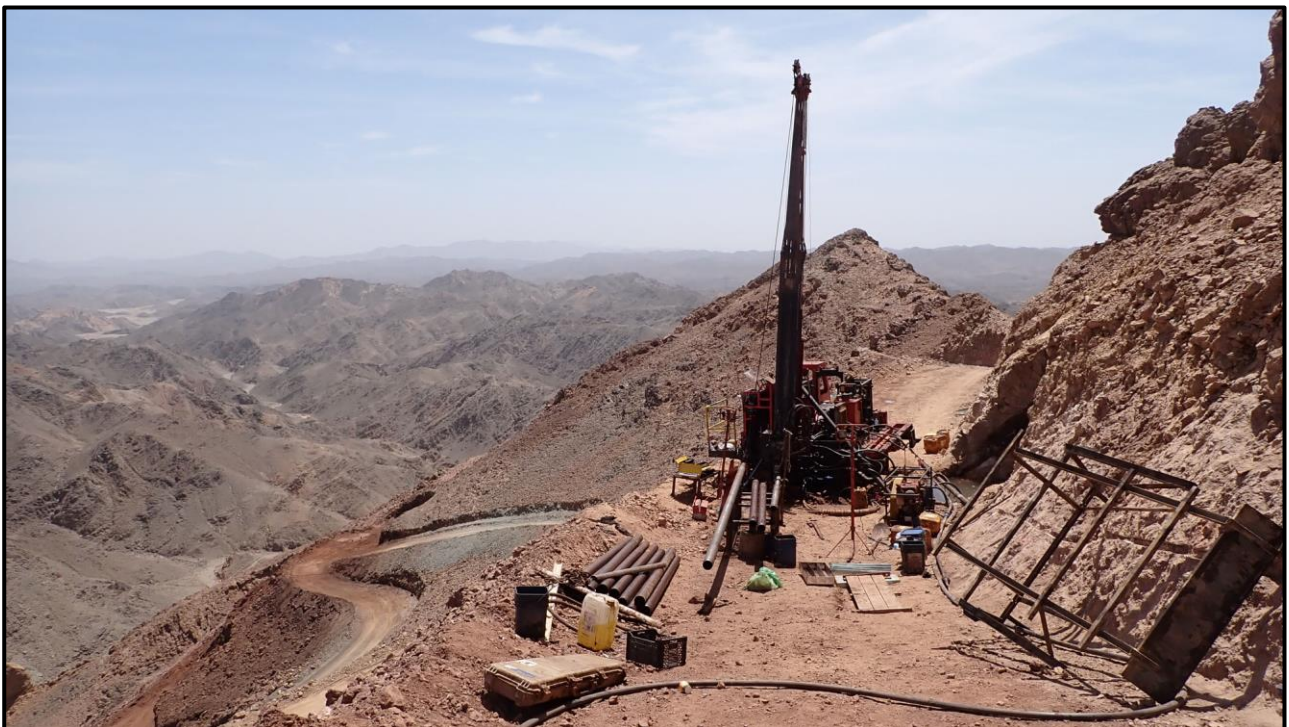
Figure 3: Drill rig set up on hole ROD-078; the ROD-077 pad is behind, below and to the left of the drill rig
