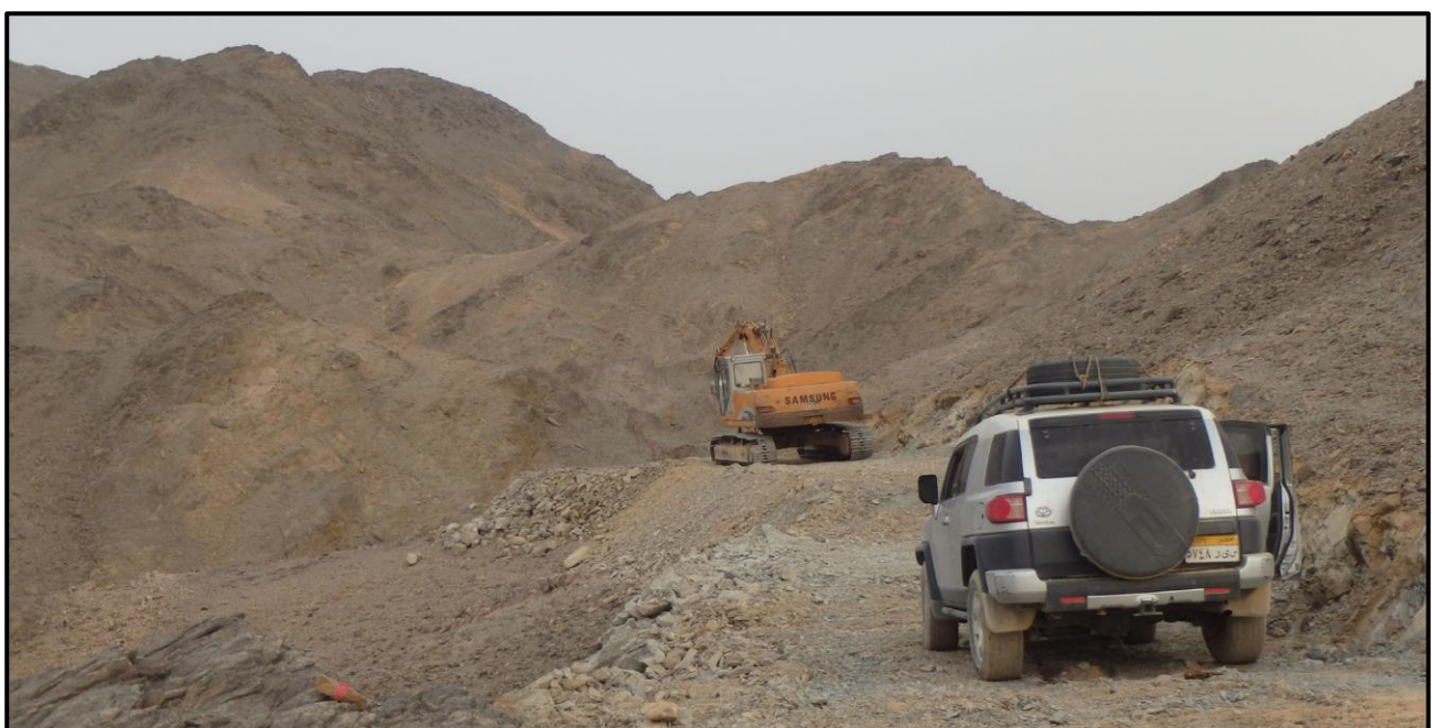
Figure 5: Rodruin access road head, as of April 13, 2018 (Rodruin is located behind the ridge above the excavator)
